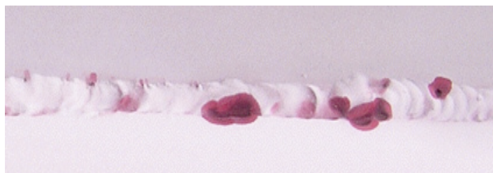
Visible penetrant indications of porosity on weld and stress cracks on metal clamp.
